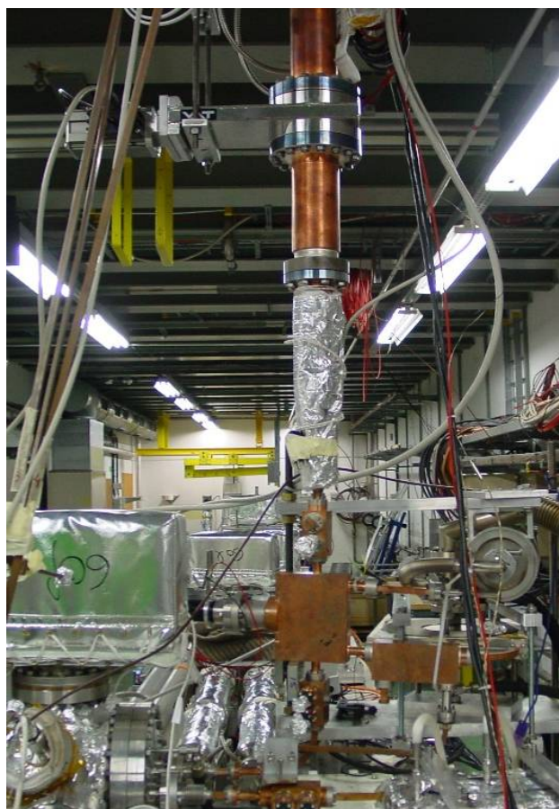
Figure 5: Quasi-optical rf waveguide vacuum valve, installed at the down-stream end of the CTF3 high-power transmission line before the 30 GHz test stand, is shown at the top. The test stand waveguide network and accelerating structure vacuum tank are also visible at the bottom.
