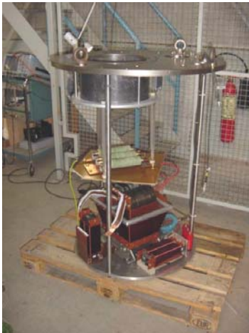
FIGURE 8 Load resistors and pulse transformer
